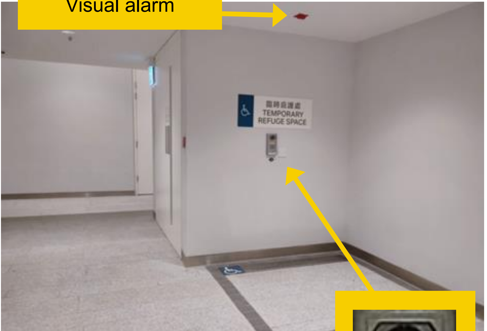
Temporary Refuge Space
